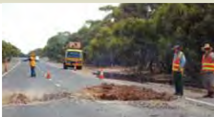
Damage to road near Ouyen
